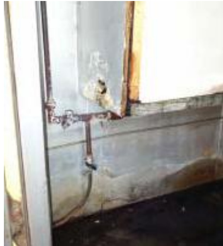
Figure 9.18 Leaking water lines
