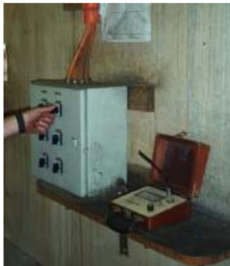
Figure 11.02. Moisture probe and a rotary switch used with a portable moisture meter. The board is connected to probes in each rack in the kiln
