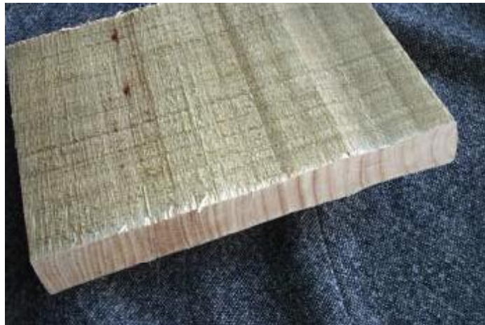
Figure 10.01. Collapse on the end and surface of a board
