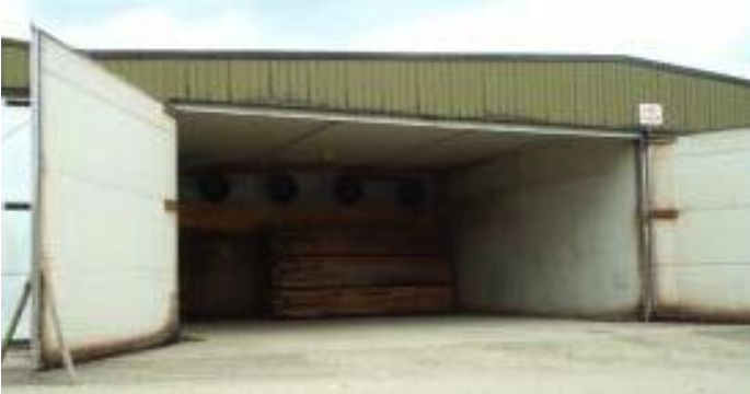
Figure 9.08. An older small conventional batch predryer
