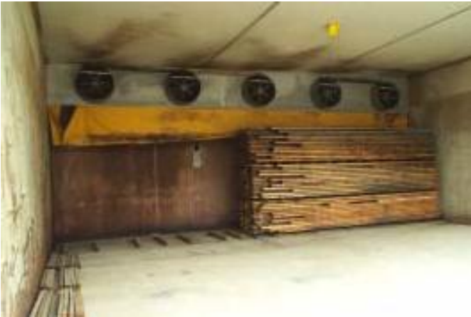
Figure 9.09. Fans and baffles in an older small conventional batch predryer
