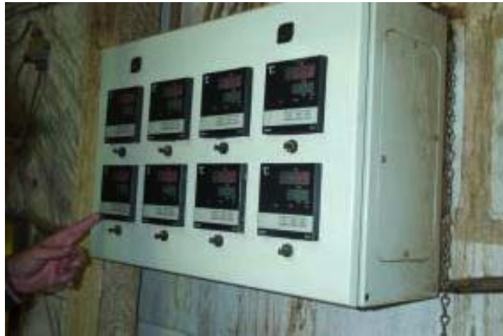
Figure 11.08. The monitoring unit for resistance moisture sensors connected to each stack in the kiln
