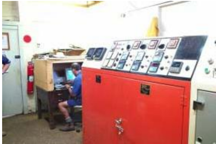
Figure 11.10. Kiln and predryer control equipment
