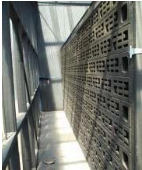
Figure 9.14. Breeze blocks provide thermal mass and an air diffuser in small greenhouse type unit
