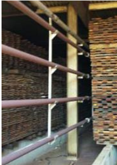
Figure 9.07. Reheating coils in a large constant condition batch predryer
