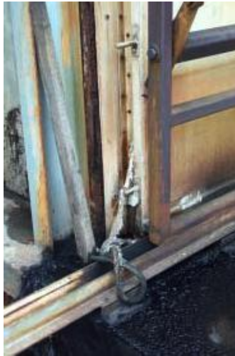
Figure 10.06 Broken door seal releases steam
