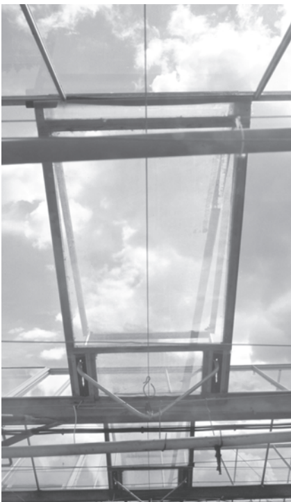
Insect pests can enter through roof vents; these should be screened as well
