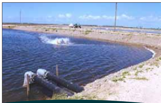
Figure 4.4 Filter screens or 'socks' installed on pond outlet pipes
