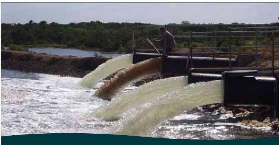
Figure 2.8 Pumping water into a reservoir
