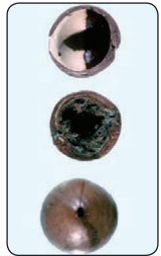
Range of damage – internal damage (top and centre), entry hole (lower)
